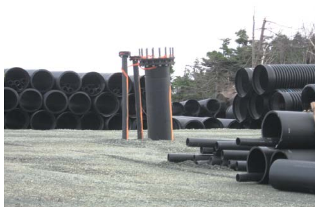
Methane Gas Flare - Robin Hood Bay Landfill site. Photo: City of St. John's.
